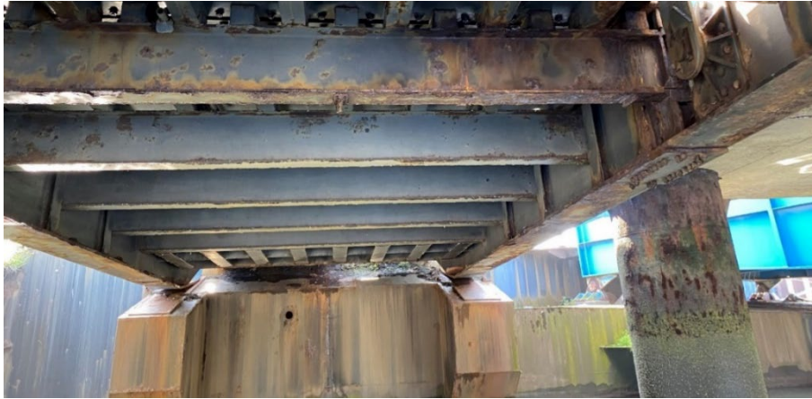
Figure 3.7 : Highly Corroded Cross Girder at Pontoon End.
