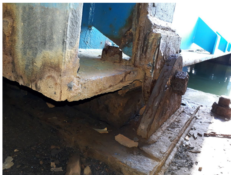
Figure 4.14 : Existing condition of bearings at the shore end.
