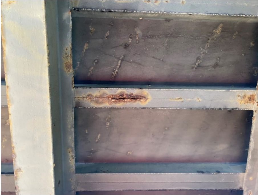
Figure 3.5 : Deck Soffit – Corrosion at Strip Locations.
