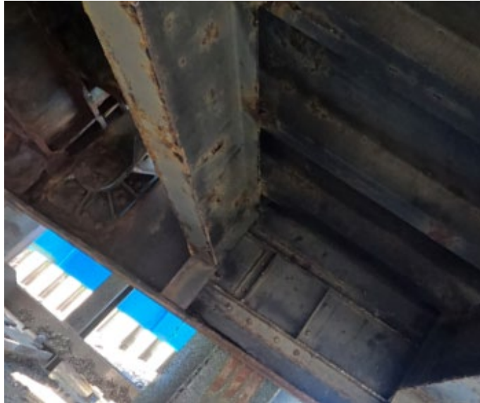
Figure 7.1 : Initial Condition of the Cross Girder and Longitudinal Stiffeners.
