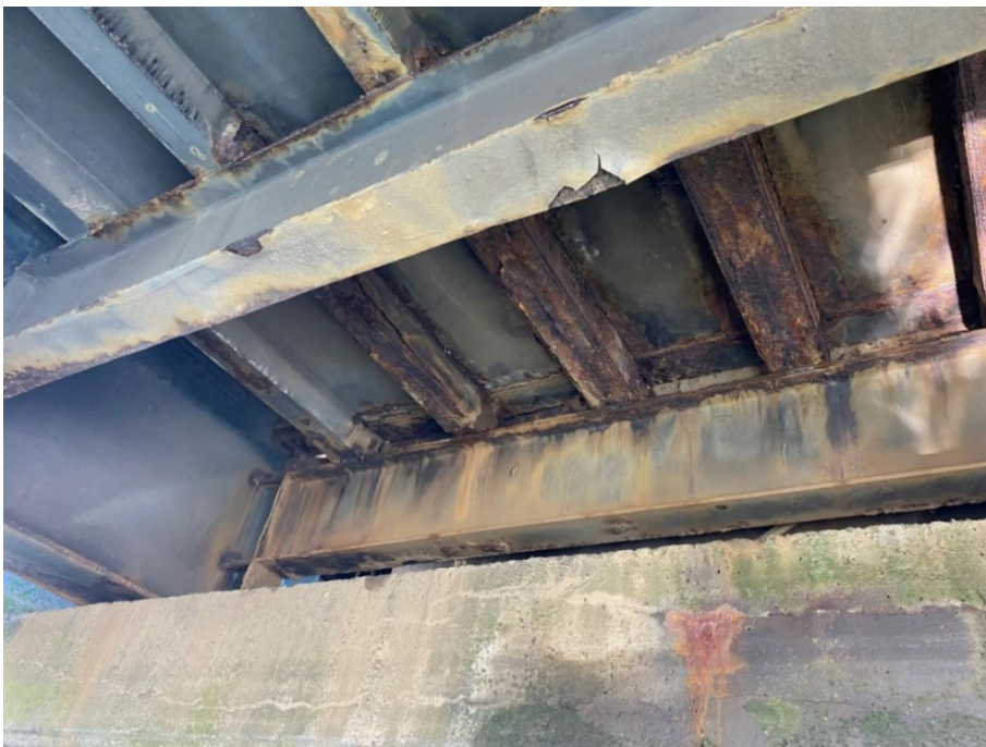
Figure 3.6 : Highly Corroded Longitudinal Stiffeners and Moderate Corrosion on Cross Girders at Abutment End.
