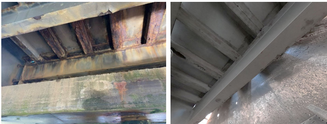
Figure 3.13 : General corrosion of box section longitudinal stiffeners.
