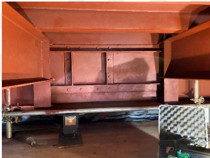
Figure 7.2 : Blasted and Shop Primed Condition of the Cross Girder and Longitudinal Stiffeners.
