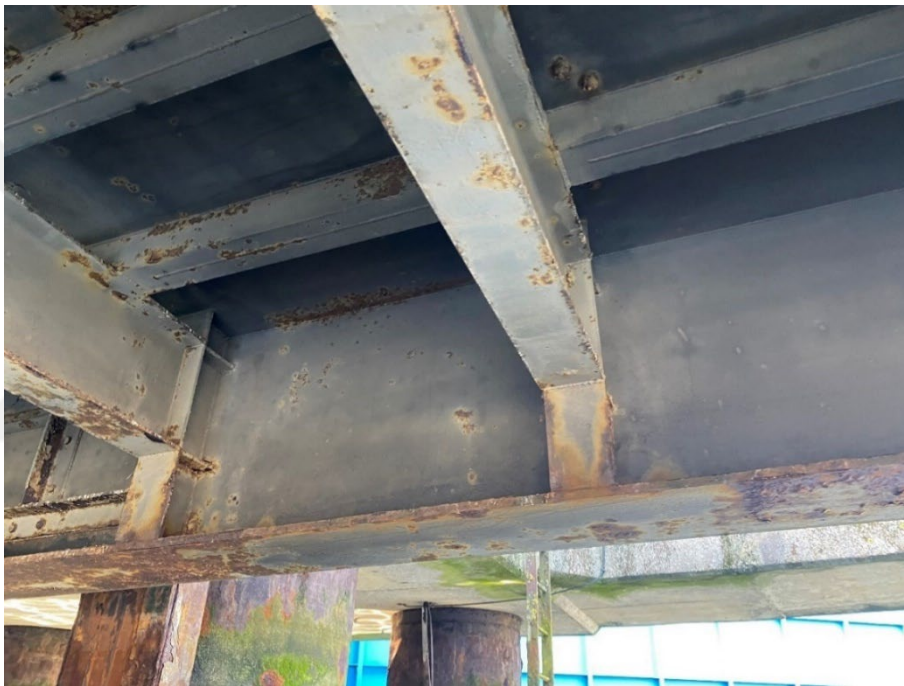
Figure 3.8 : General Attack Corrosion at Bottom Flange of Main Girder and Localised Corrosion at Cross Girders – Extension Area.
