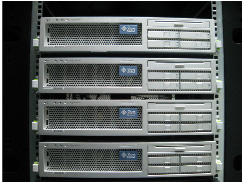
Figure 12. New four node processing server setup
