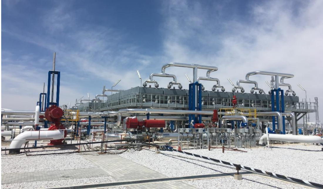
Figure 3.16: Tuz Lake natural gas storage facility (Url-17).
