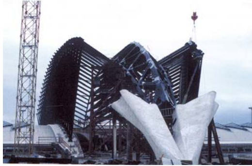
Terminal building, Railway Station at Satolas Airport, 1994, S.Calatrava, TGV Binası. Merkezdeki kemer omurga ve yan payandalar
