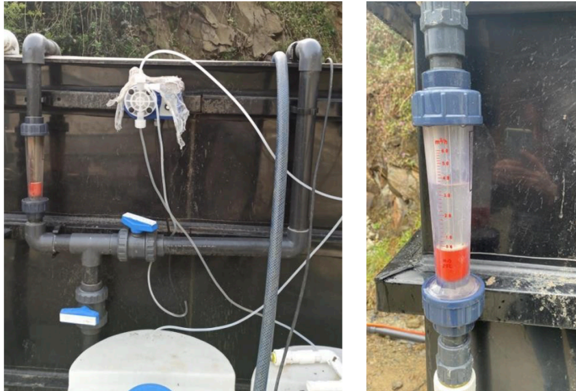
Figure 2.11 : The recirculation line and flowmeters of the pilot scale IFAS MBR system.
