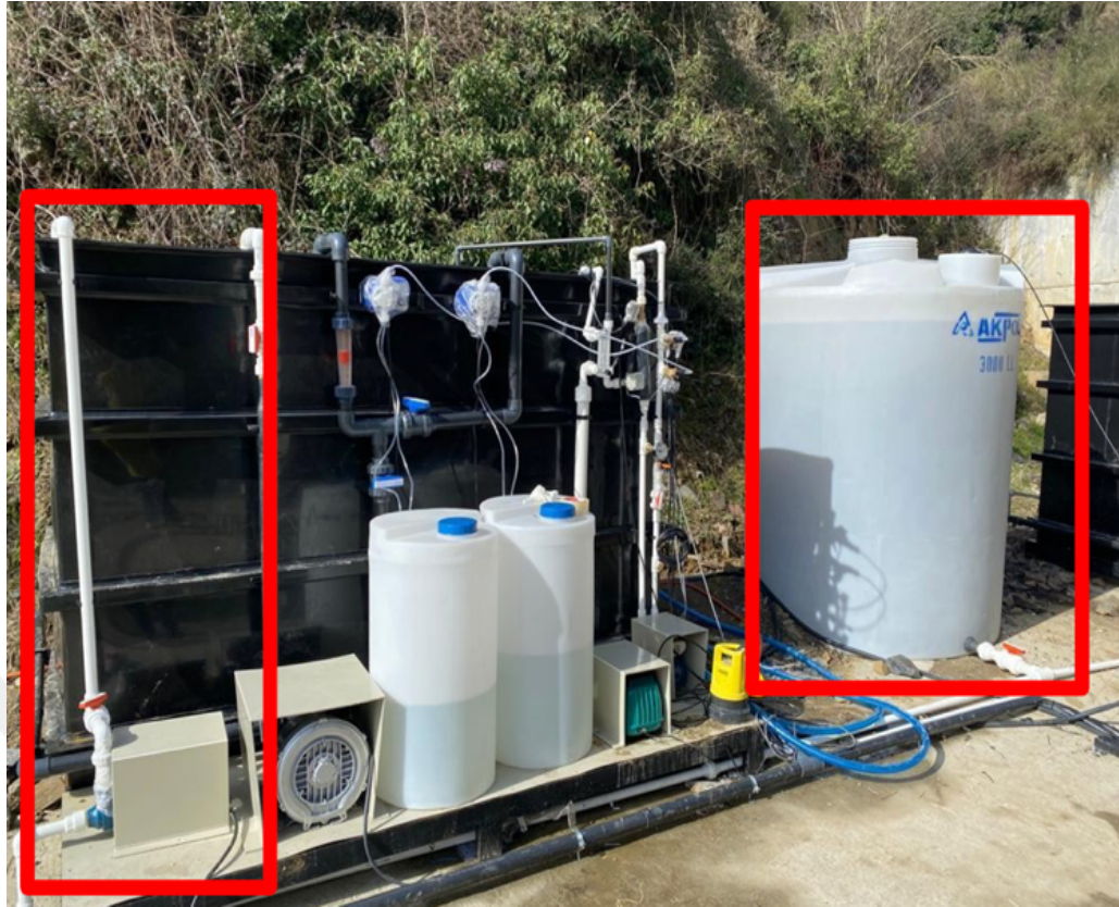
Figure 2.9 : The feed pump of the pilot scale IFAS MBR system.
