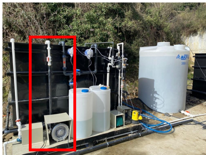
Figure 2.10 : The aeration line of the pilot scale IFAS MBR system.
