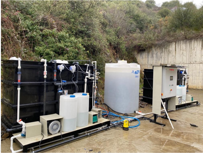
Figure 2.4 : The general overview of the pilot scale IFAS MBR systems.
