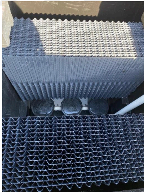
Figure 2.5 : IFAS carrier media located in aeration tank.
