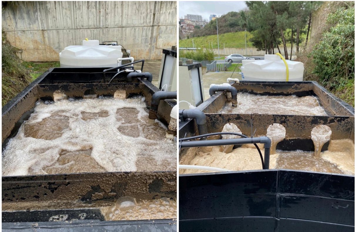
Figure 2.6 : The general appearance of the pilot scale IFAS MBR system after the seed sludge has been filled to the reactors.
