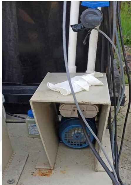
Figure 2.15 : The vacuum pump of the pilot scale IFAS MBR system
