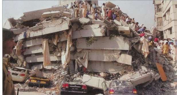
Figure 3.3 : Collapse earthquake (Nasril, 2011)
