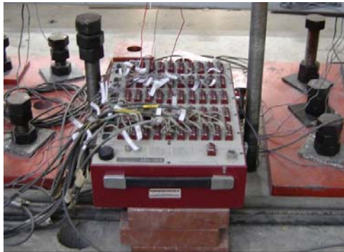
Figure 4.23: Switch Box Used on Test Site
