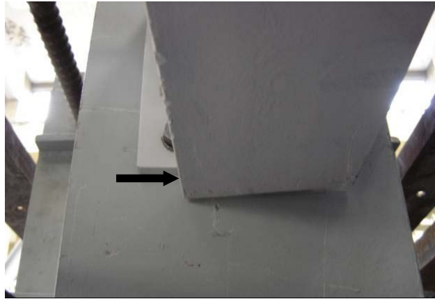
Figure 7.12: Movement of the North End of the Top Beam (Specimen BF-H, Cycle 32 and Top Disp. of 81.81mm)
