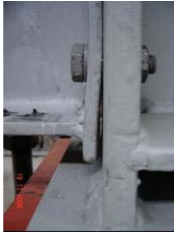
Figure A.5: Gap between the Beam End Plate and Column Flange (Specimen BF-F, Cycle 19 and Top Disp. of 23.20mm)
