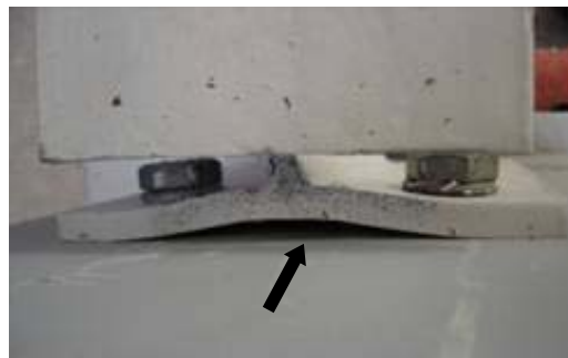
Figure 7.5: Gap between the Beam End Plate and Column Flange (Specimen BF-H, Cycle 25 and Top Disp. of 46.79mm)
