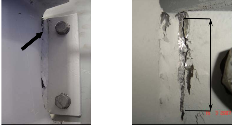
Figure 7.9: End Plate Fracture (Specimen BF-H, Cycle 31 and Top Disp. of 81.81mm)
