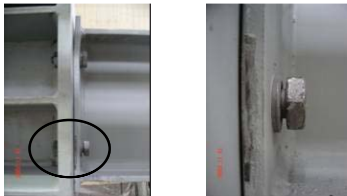
Figure A.6: Failure Bolt at the East Side of the Bottom Bolt-Row (Specimen BF-F, Cycle 23 and Top Disp. of -34.35mm)
