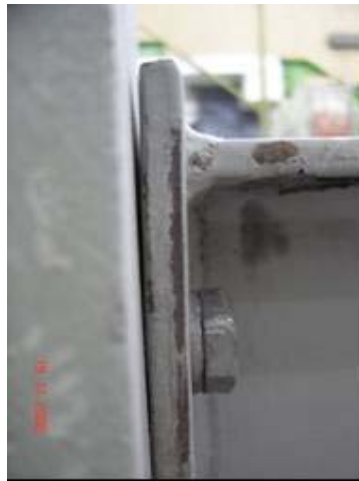
Figure A.4: Gap between the Beam End Plate and Column Flange (Specimen BF-F, Cycle 10 and Top Disp. of -5.74mm)
