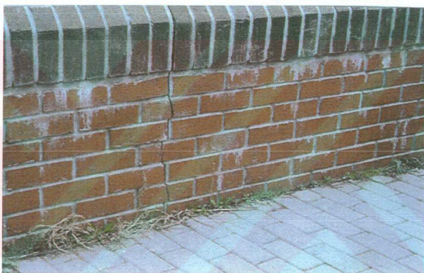
Fig. 3.18 Crack Caused By Grouting Pressure
