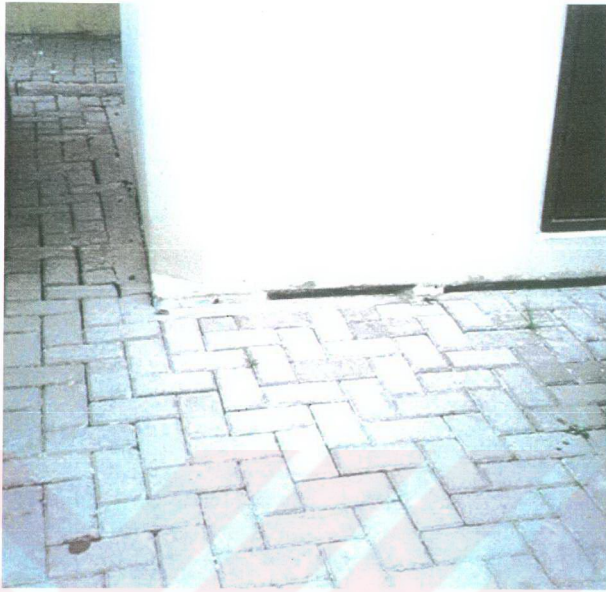
Fig. 3.16 Swelling under The Transformer Building Right Behind The General Directorate Building
