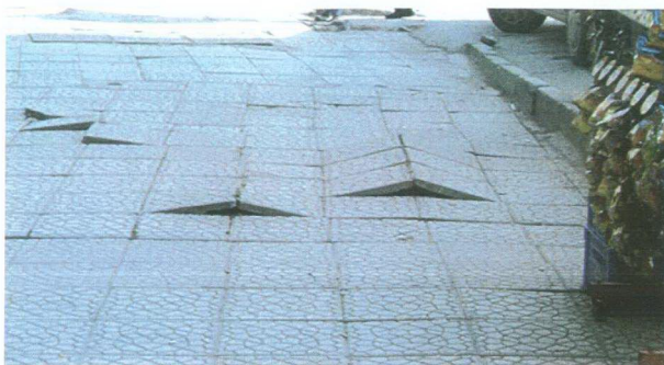
Fig. 3.17 Risen Pavement Stones
