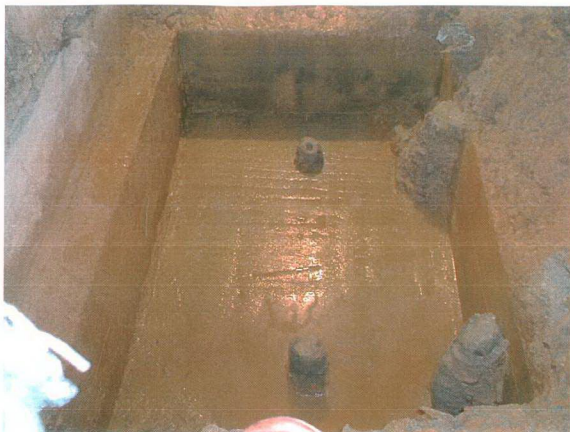
Fig. 3.22 Uncovered Section of Floor
