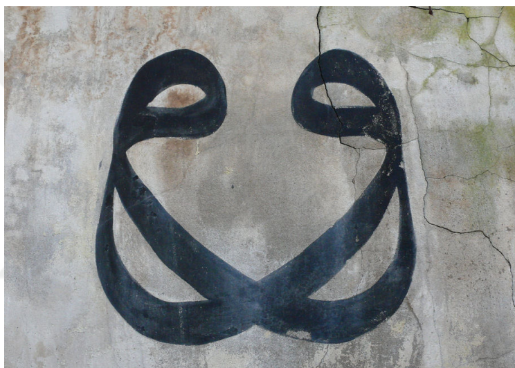
Figure 5.1 : Çifte Vav . (Symmetrical letters of V [ﺹ] symbolizing vahdet (unity). The surviving calligraphy on the wall of Kadirîhâne after the fire. Photography by Caner Cangül [2009] before the restoration).
