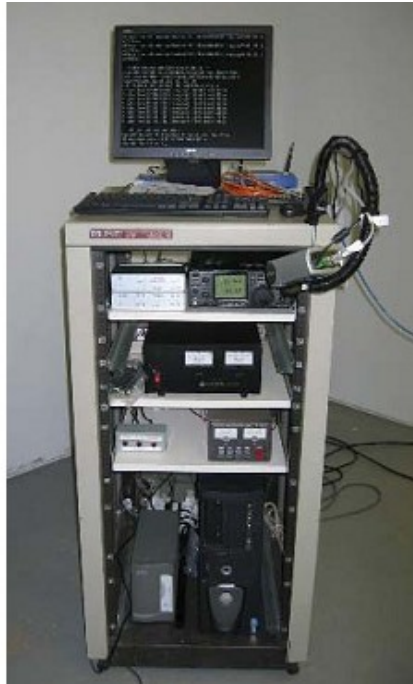
Figure 4.14 : Fairbanks Ground Station Equipment Rack.
