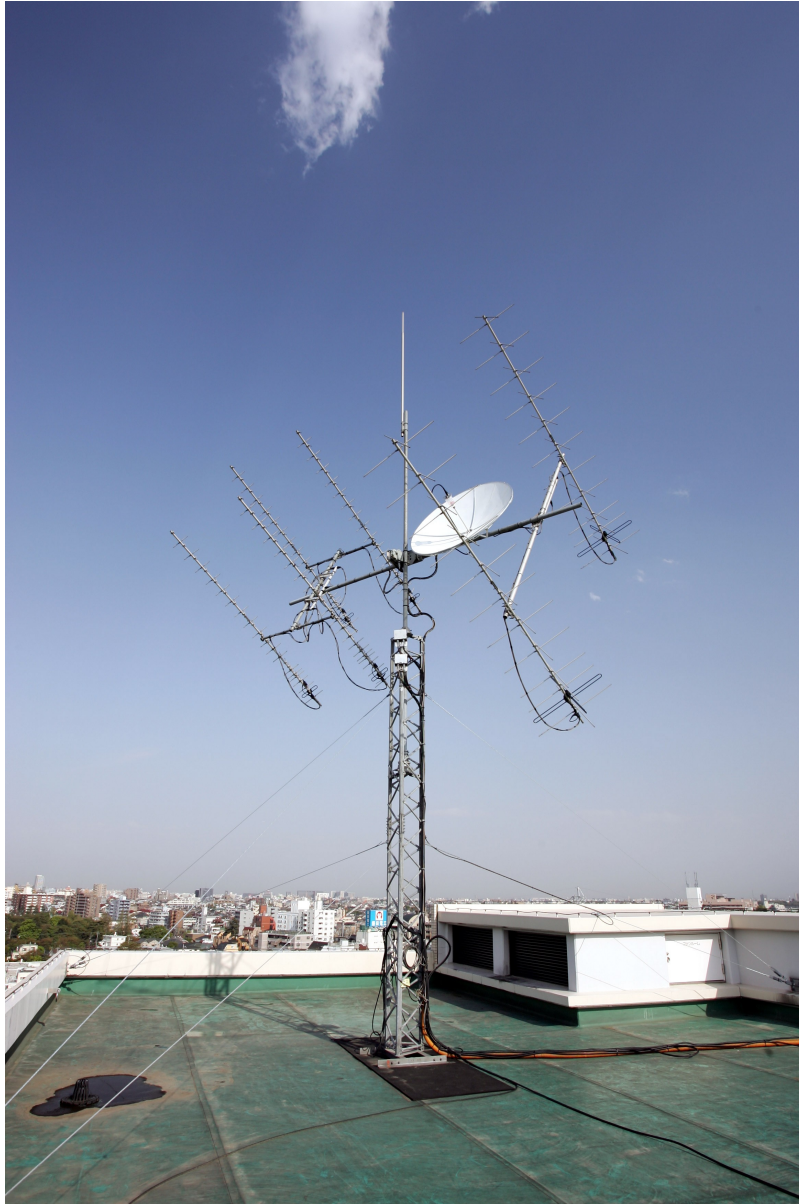
Figure 4.25 : TiTech Ground Station antennas.
