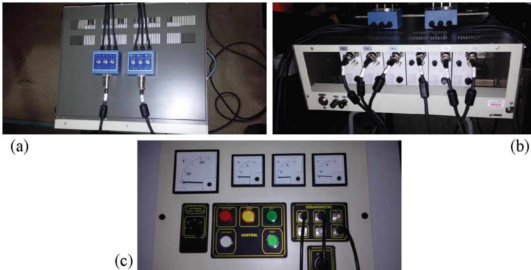
Figure 3.16 : Electrical equipment installation: (a) Calibration boxes, (b) Separation of the force and moment components, (c) Control panel.
