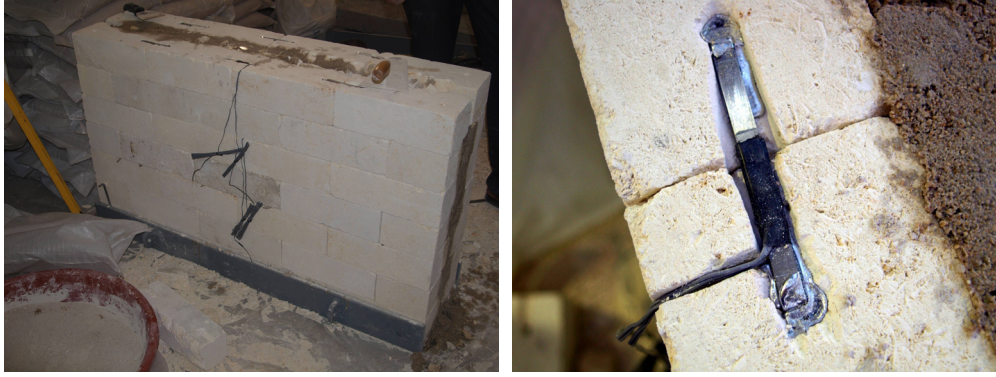
Figure 3.10 : Fitting of the instrumented cramps.
