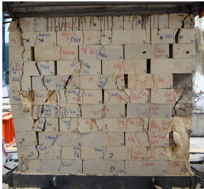
Figure C.131 : Northern face of M-50 specimen after the test.
