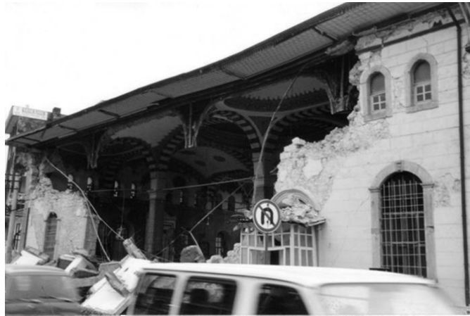
Figure 1.2 : Mosque damaged by the 1999 Marmara earthquake (Ilki et al., 2006).
