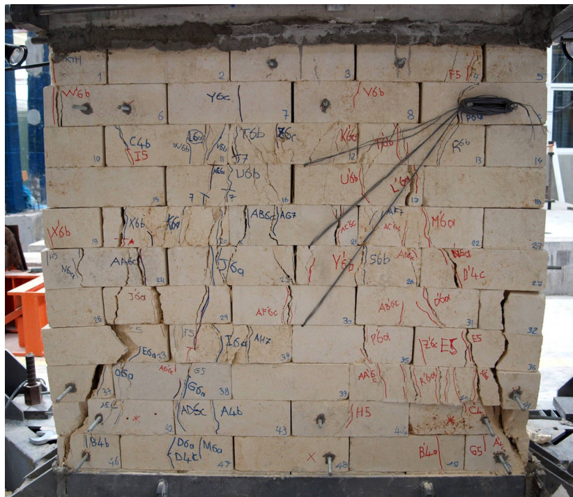
Figure C.42 : Cycle 8, North face of M-50-C after 1.50% drift ratio.
