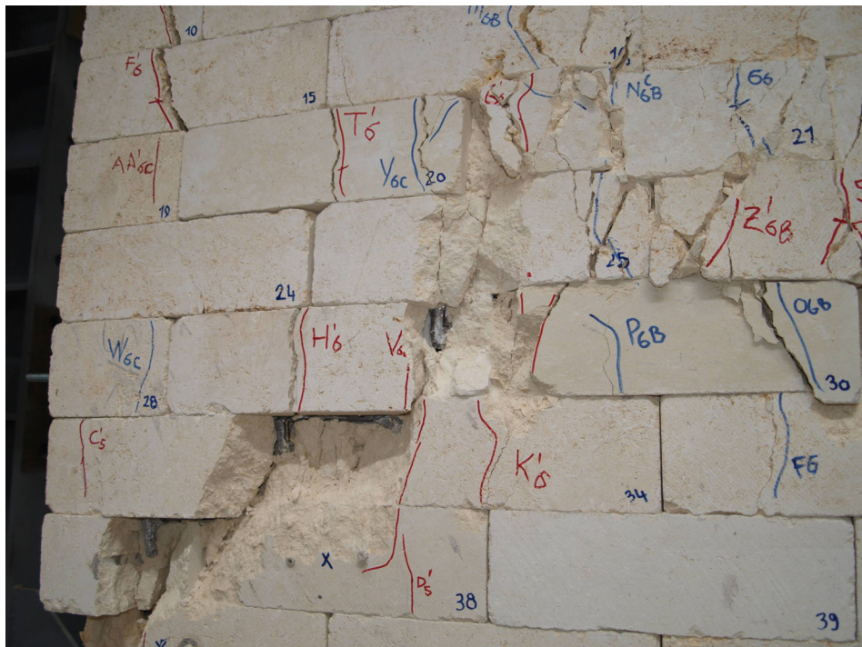
Figure C.74 : Damage in the vicinity of cramp anchors, M-75-C.
