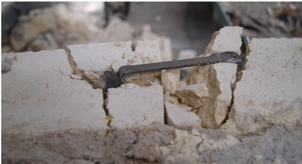
Figure C.45 : Damage in the vicinity of cramp anchors, M-50-C.
