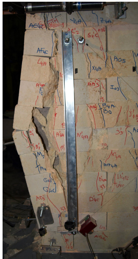
Figure C.99 : Cycle 6a, Buckling of the vertical column after 1.00% drift ratio.
