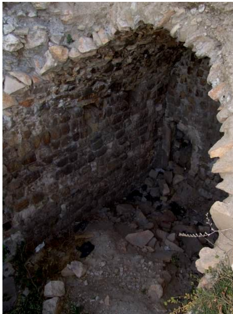
Figure 2.255 : The collapsed vault of the VM3 aiwan – looking northwest.
