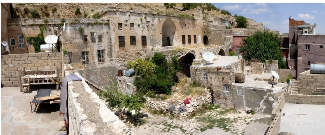
Figure 2.70 : The main courtyard, the collapsed VM3 aiwan and the upper layer – looking northeast from the IIIUt terrace.
