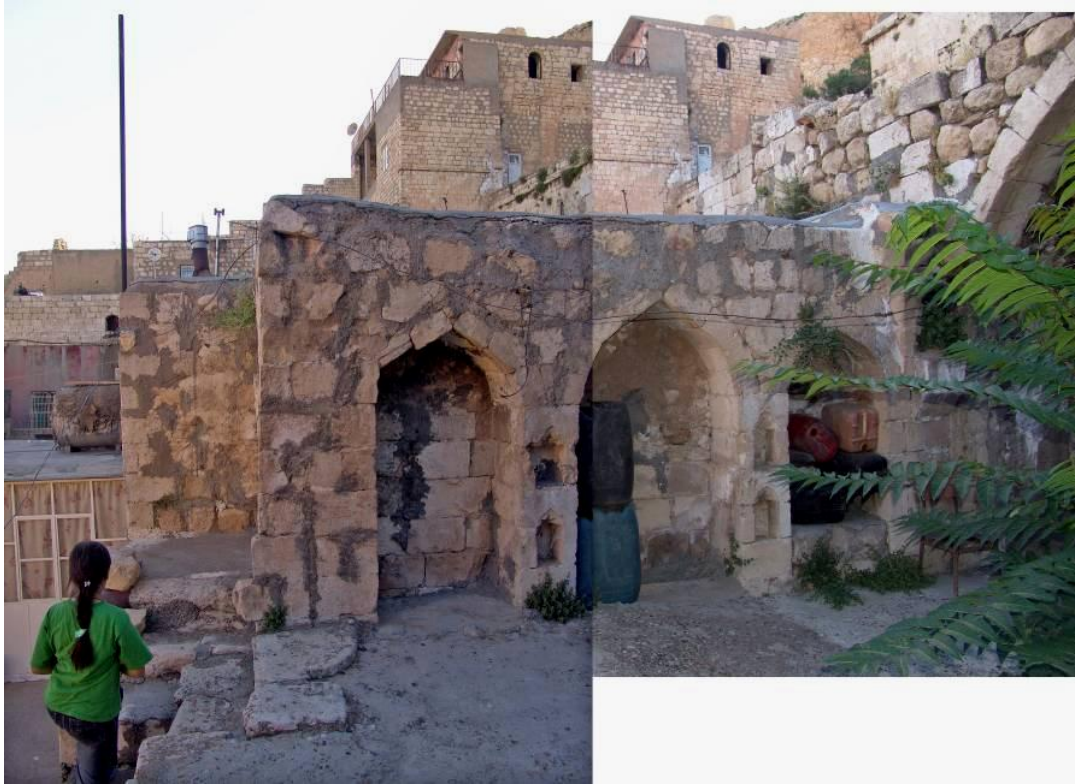
Figure 2.268 : The western wall of the VM6 terrace/collapsed volume.
