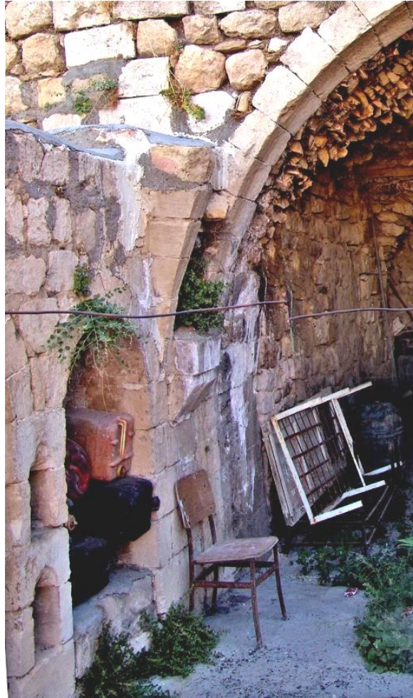
Figure 2.271 : The vault impost between the VM4 volume and the collapsed VM6 volume.
