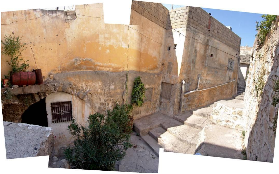
Figure 2.79 : The collapsed IIL2 volume the main entrance to the internal street – panoramic from the south towards the west – looking from the IM3 entrance.
