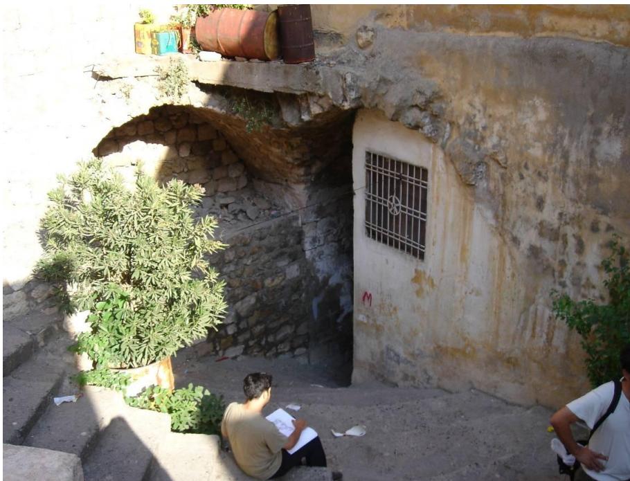
Figure 2.82 : The collapsed groin vault IIL2, where the staircase rises to almost the lower level of the groin vault – looking southeast from the south of Block-V.
