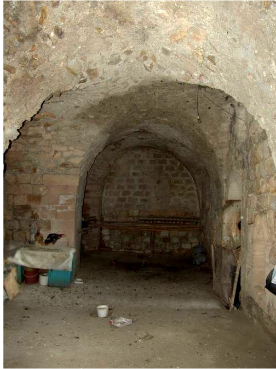
Figure 2.240 : The storage system constituting the north of Block-VI – looking east.
