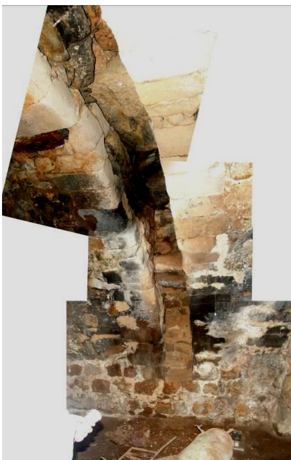
Figure 2.308 : The collapsed arch of the ILL3 volume – looking southwest.
