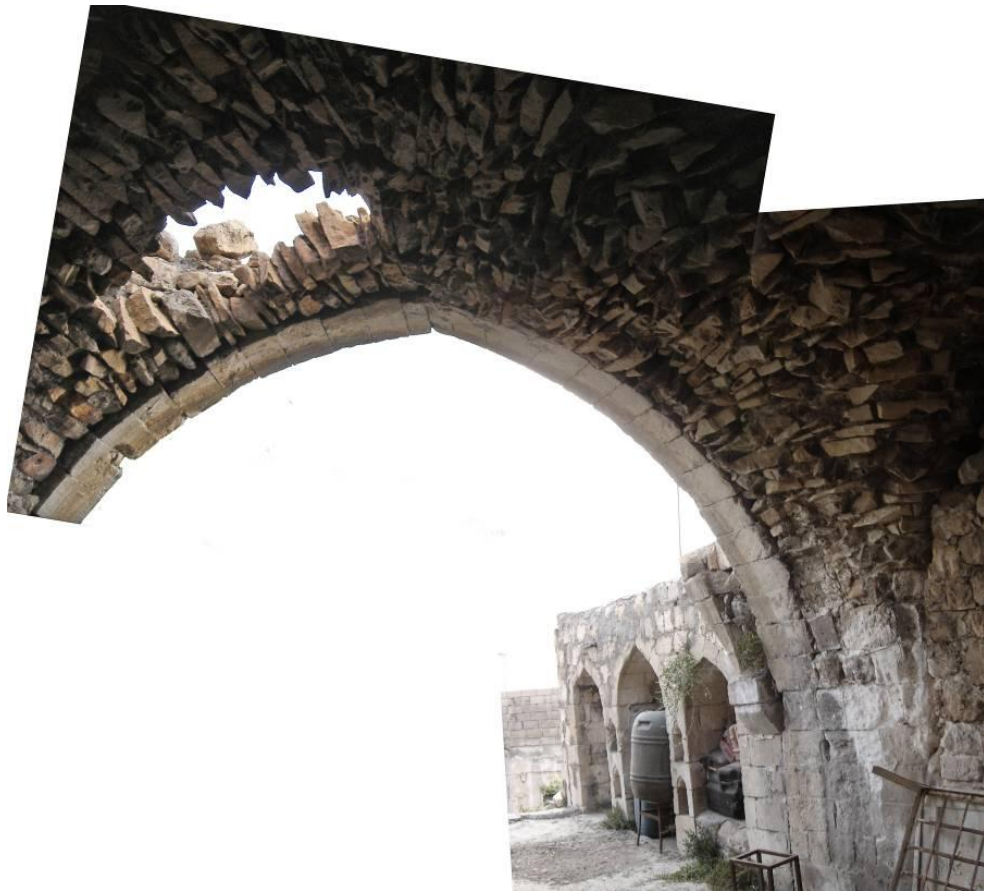
Figure 2.270 : The near-collapsed vault of VM6 – looking south.
