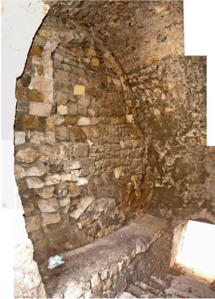
Figure 2.80 : The current entrance staircase volume (IIL1) to the main courtyard – looking southeast towards the collapsed wall between IL1 and IIL1.
