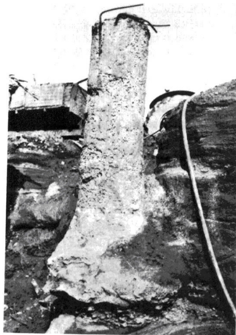
Figure 3.1: Bulbous projection on pile shaft caused by overbreak. (Flaming, 1992)
