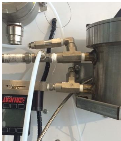
Figure 5.9: Inlet (upper) and outlet (lower) of the reactor.
