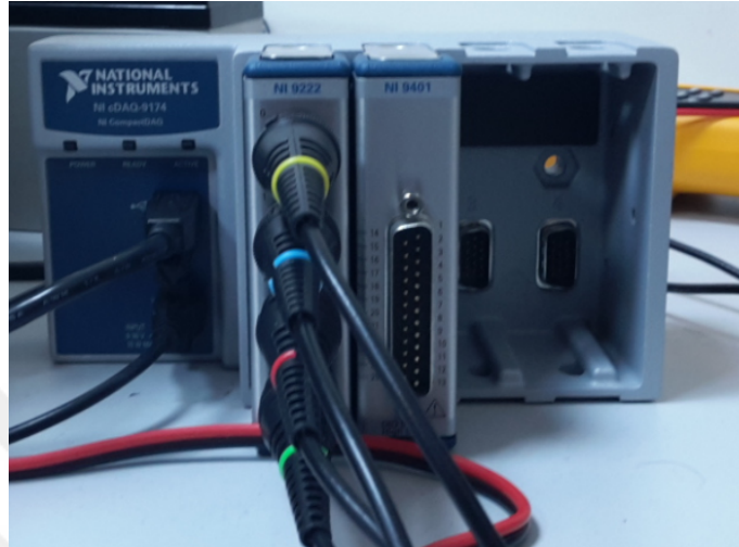
Figure 4.3 : Mounted NI CDAQ modules.
