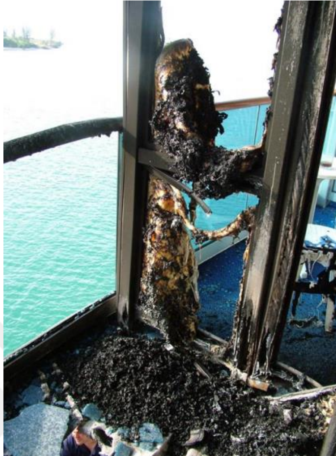
Figure 5.3 : Melted polycarbonate partition of Star Princess.
