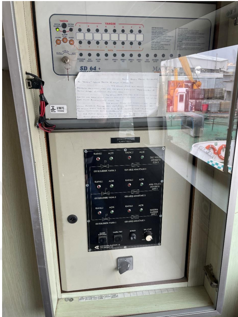
Figure H.5 : Control panel of fire sprinklers and valves in SH-SUTLUCE.
