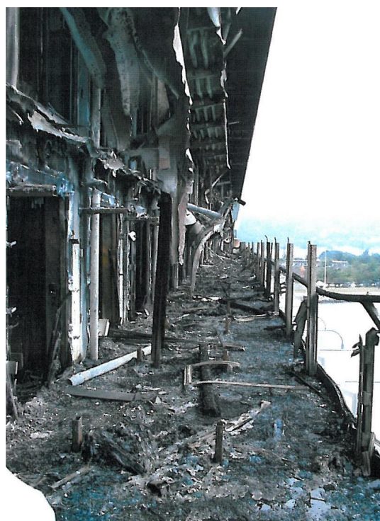
Figure 5.2 : Melted aluminium structure of Star Princess.
