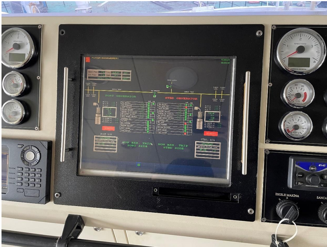
Figure H.3 : Fire safety control panel of SH-SUTLUCE.
