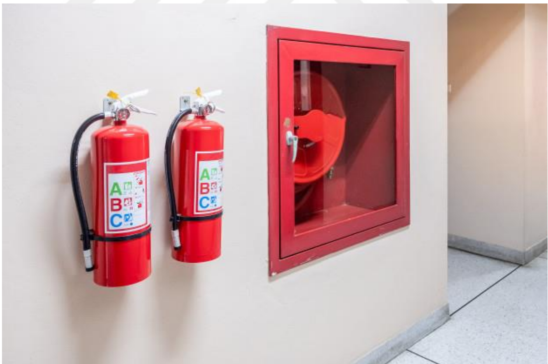
Figure B.2 : Portable fire extinguishers.
