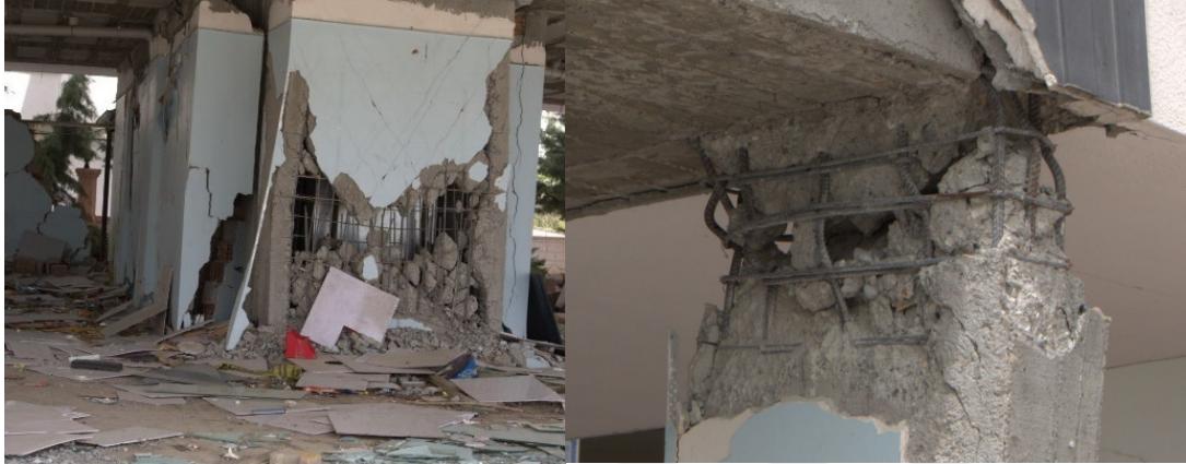
Figure 2.5 : (a) Shear walls had low quality concrete and not designed for the immense amount of shear force. (b) Damage was concentrated at the connections (Cilesizoglu, 2023).
