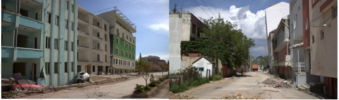
Figure 2.7 : (a) As a result of liquefaction, buildings subsided and overturned, rendering them completely uninhabitable. (b) Subsided buildings (Cilesizoglu, 2023).
