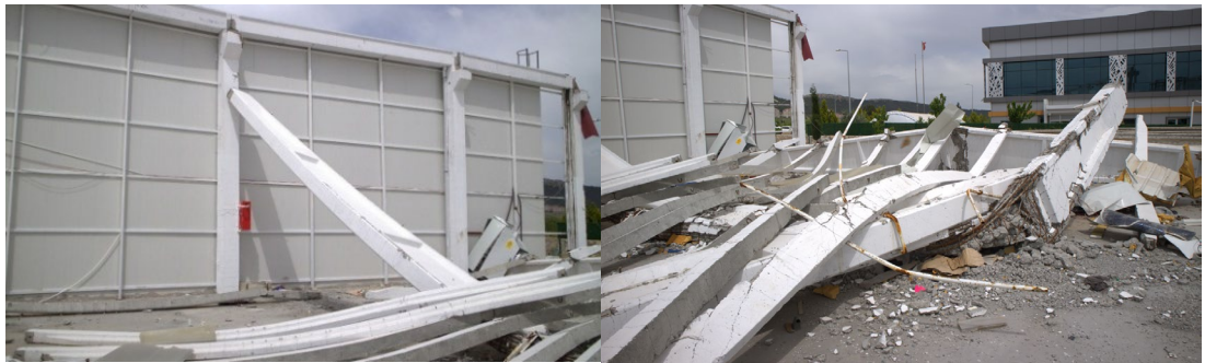
Figure 2.8 : Heavily damaged/collapsed prefabricated factory buildings on the outskirts. Connection of concrete elements was not done according to code (Cilesizoglu, 2023).
