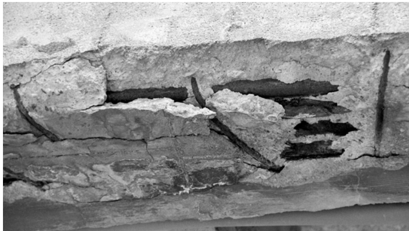
Figure 2.3 : Spalling of Concrete due Carbonation and Chloride [42]
