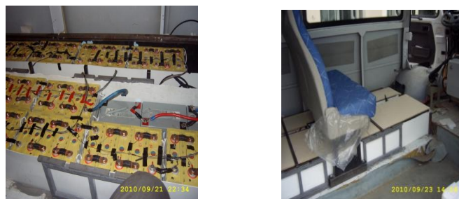
Figure 4.6 Battery Cells under Seats.
