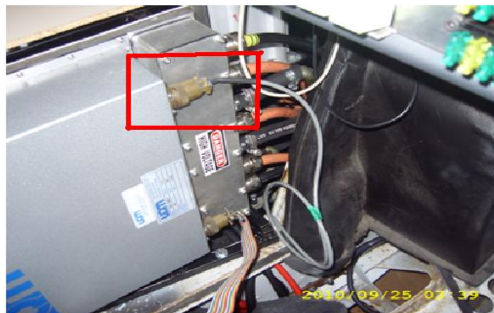
Figure 3.9: Rotor Position Cable on Controller Side.
