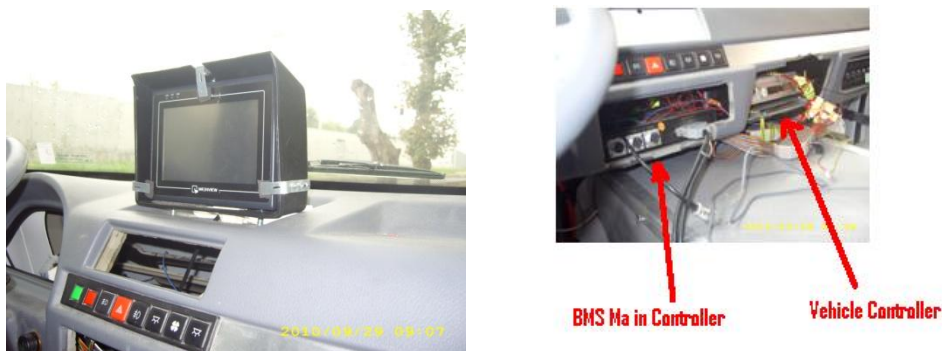
Figure 4.13: BMS Main Controller & Screen Place.
