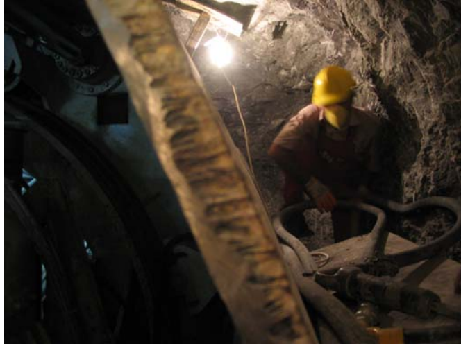
Figure 6.13 : Hand mining operation after tunnel collapse in Mavi (Blue) Tunnel.
