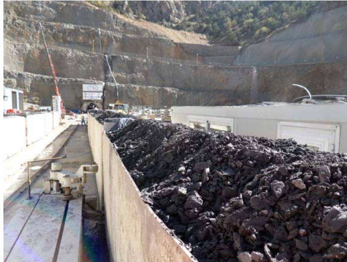
Figure 6.12 : Excavated material just before tunnel collapse.
