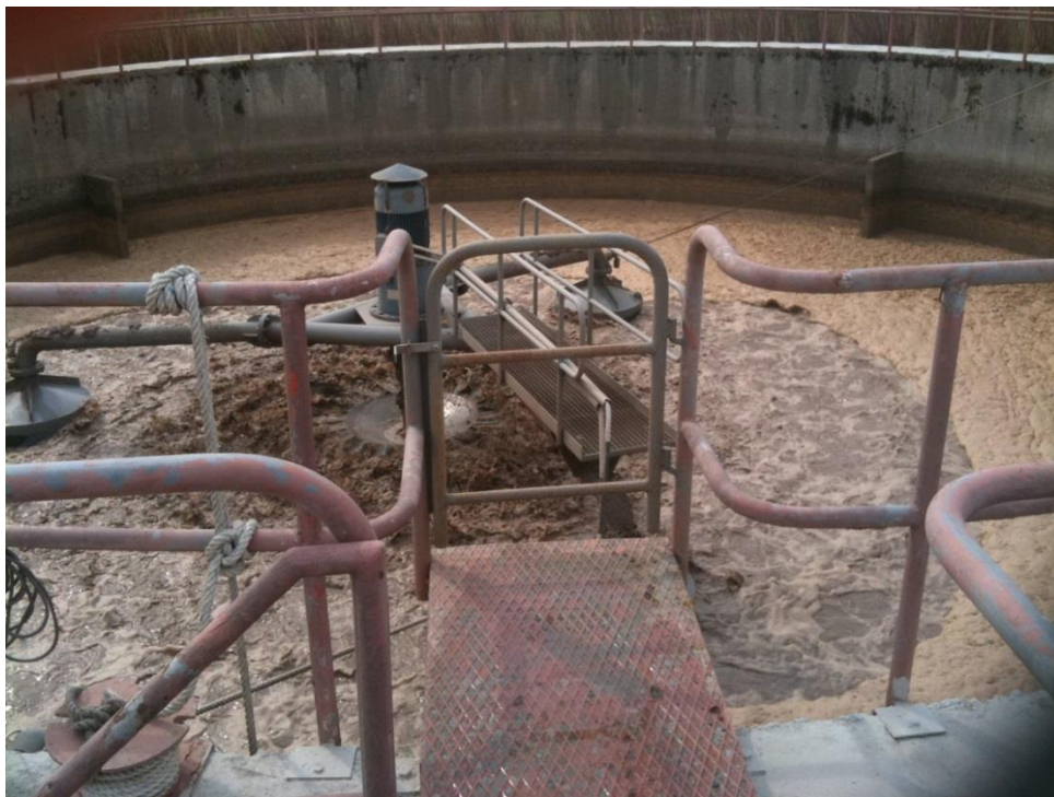
Figure 3.14. Biological Treatment Reactor (aerators in working mode).
