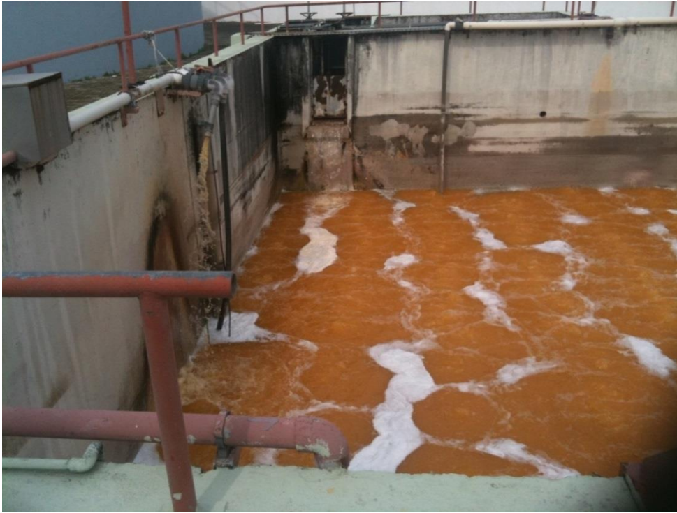
Figure 3.11. Domestic and Industrial Wastewater Entries to Mixing Pool.
