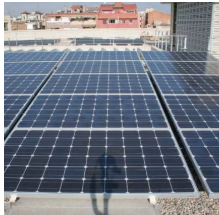
Figure 4.18: PV installation on the roof [69].
