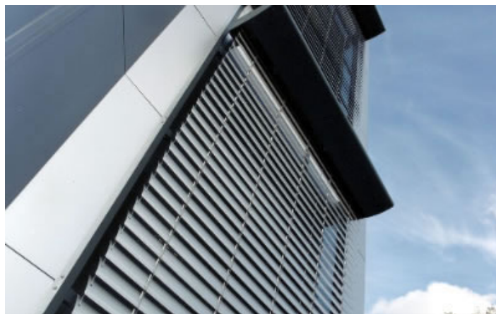
Figure 3.15: External Venetian Blinds [43].
