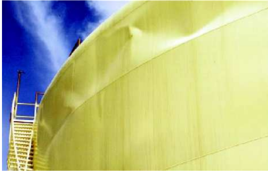
Figure 1.3: Diamond Shape Buckling (Malhotra, 2000).
