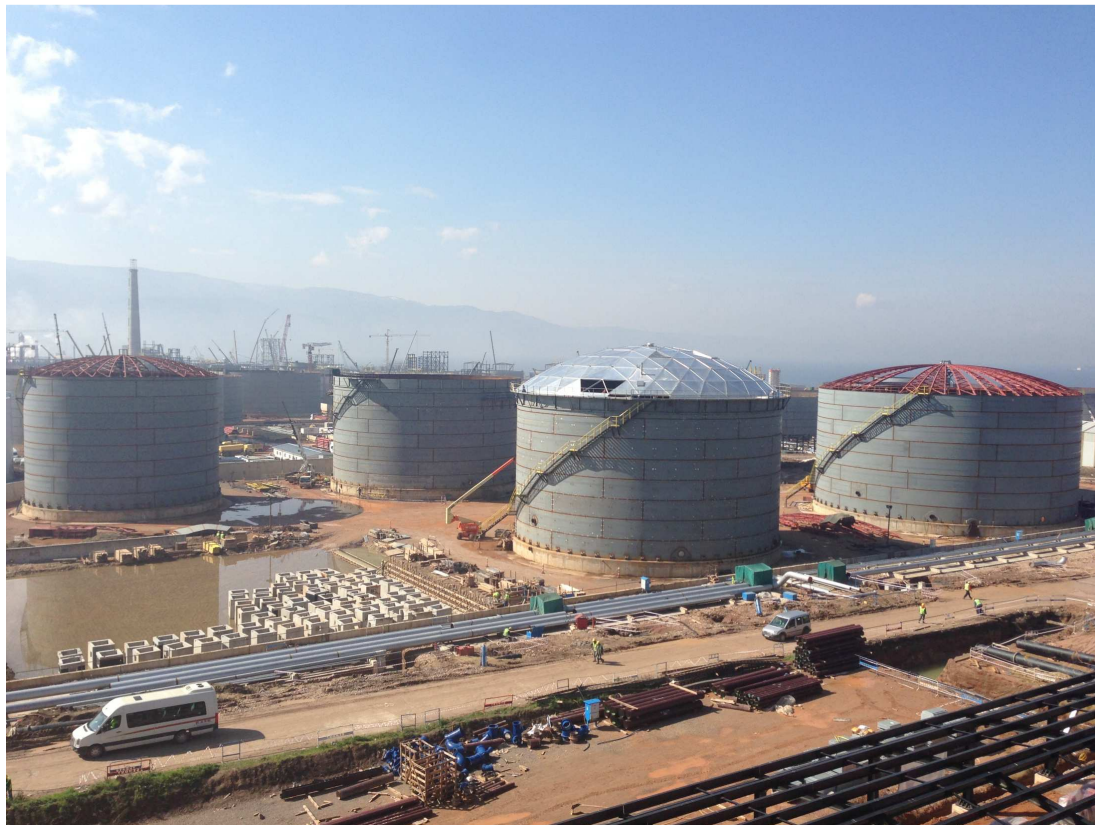
Figure 1.1: Residium Upgrading Project (TUPRAS, 2013, Personel Picture).
