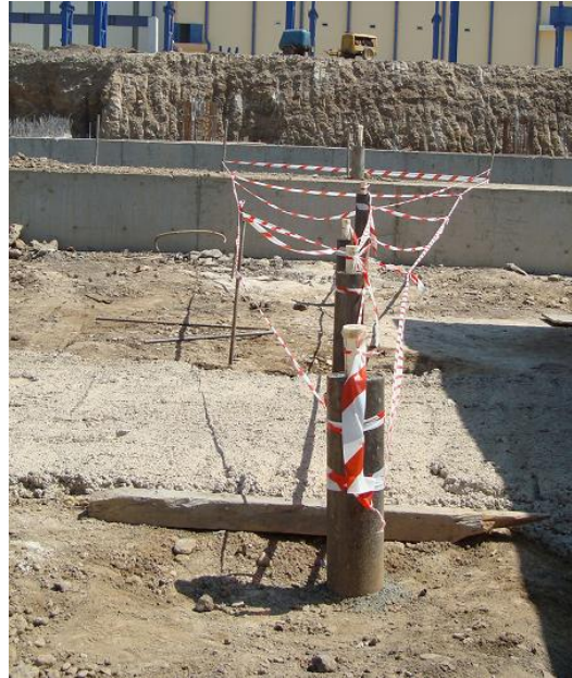
Figure 4.17: Location of the Inclinerometers behind Retaining System.
