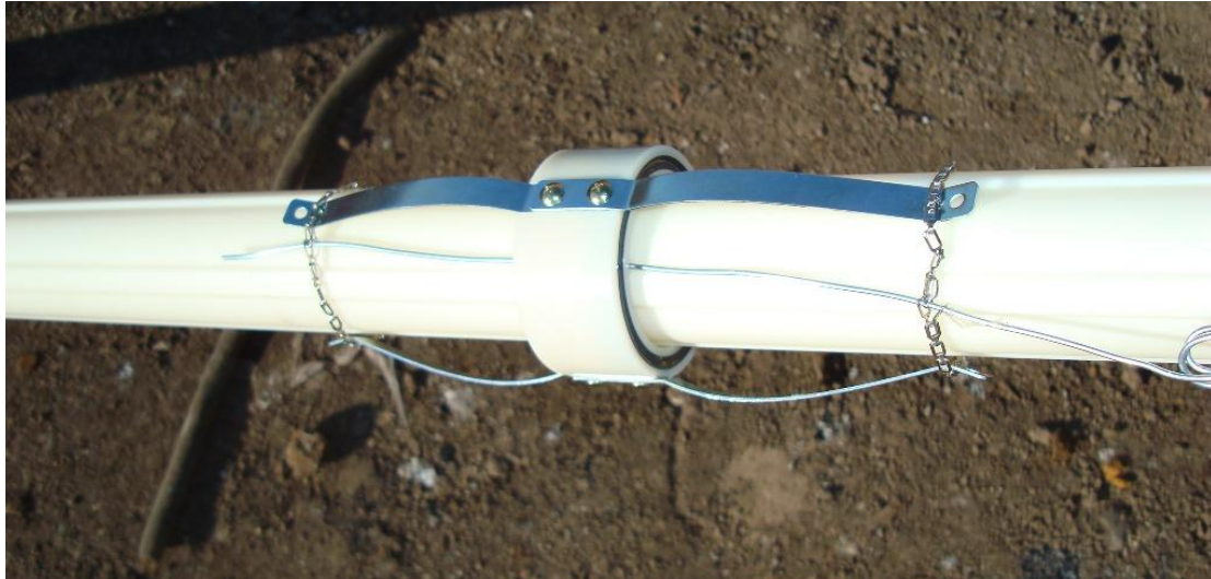
Figure 4.28: Magnets on the Inclinator Casing.
