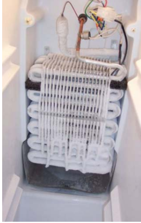
Figure 3.3: Icing on the evaporator surfaces
