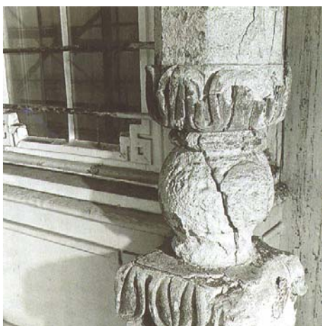
Figure 6.2- 4 Detail from a stonework affected by wet rot [56, p. 41].
