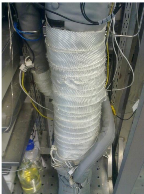
Figure 3.12 : Vaporizer with insulation.
