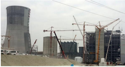
(e) Eskişehir termik santrali
