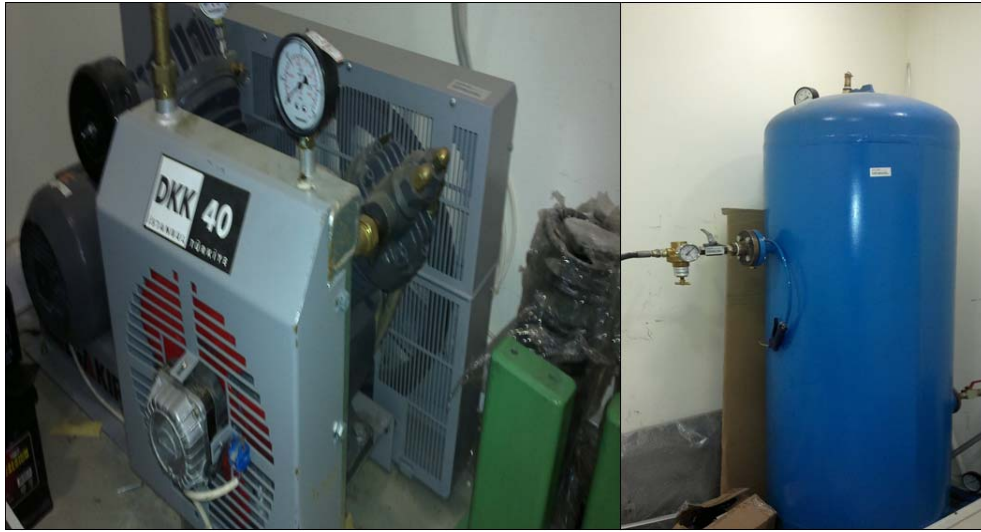
Figure 4.14 : The air compressor and the pressure tank.
